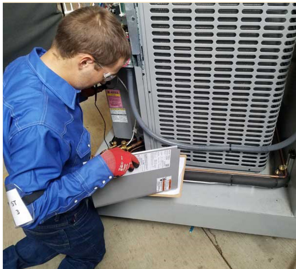
An engineer handling an A2L refrigerant unit.
