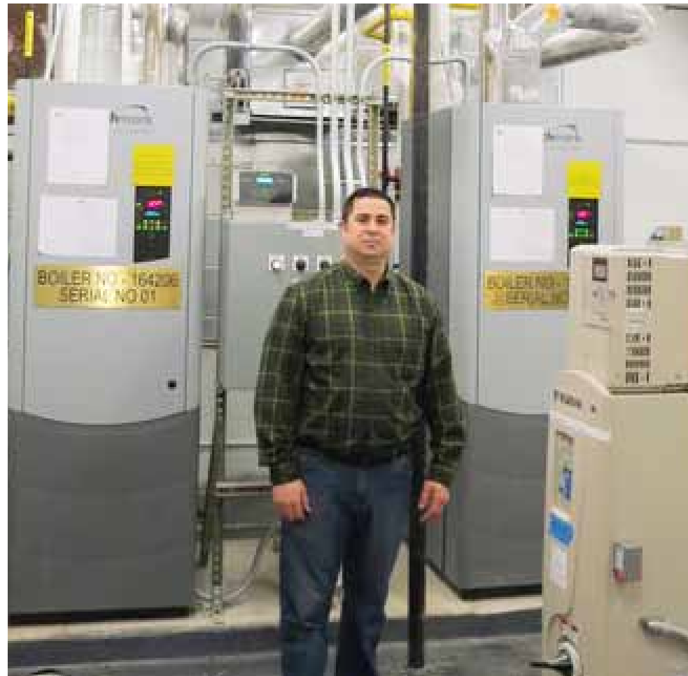
PS 51 custodian Steven Velez stands in front of new boilers.
