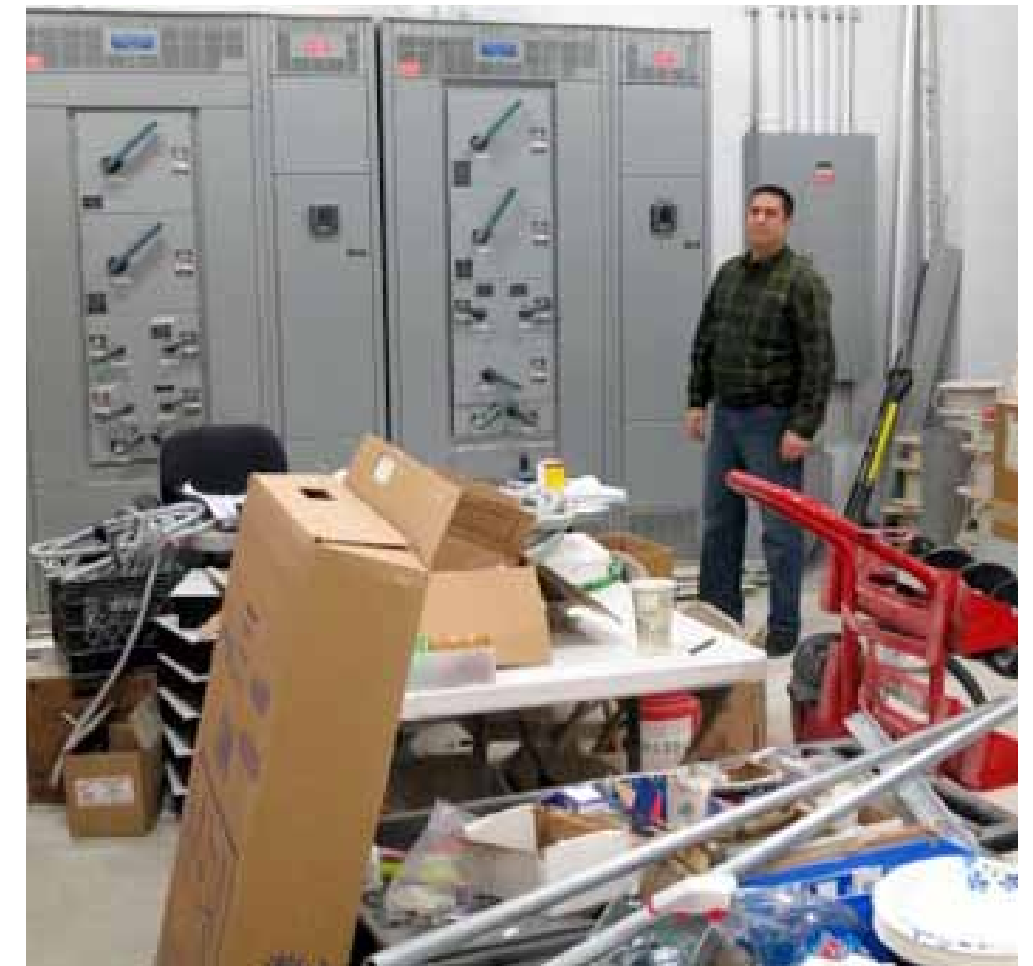
Installation work has yet to be completed inside the electrical room.
